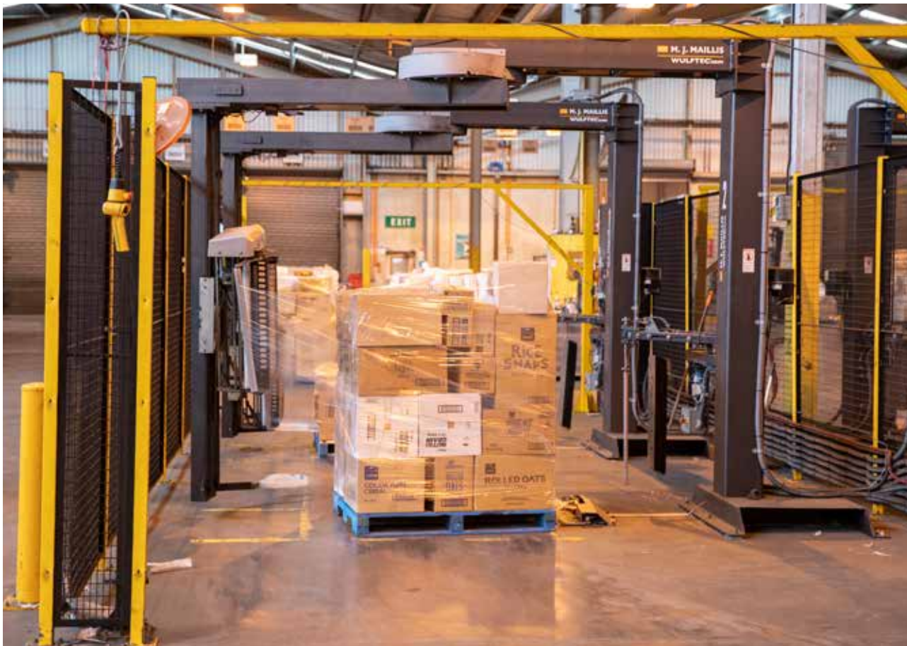
NanoWrap in action at Roma Distribution Centre
