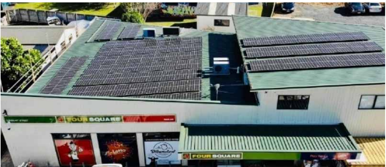
Solar panel array on Raglan Four Square
